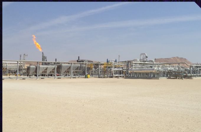
30 mmscf/d rental natural gas compression and processing facility, Oman.
