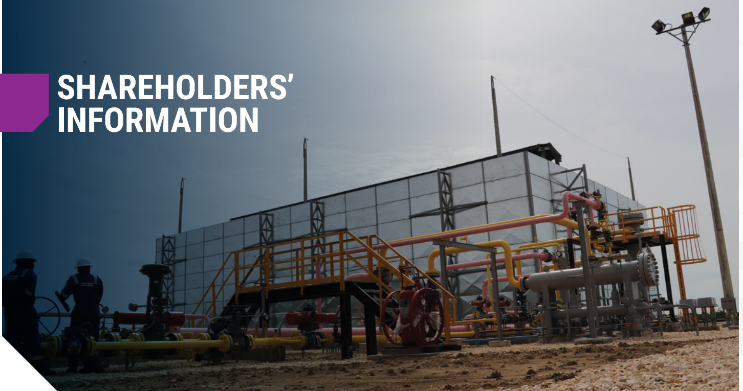
42 mmscf/d natural gas compressor station, Colombia.
