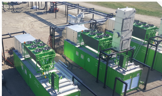
3 MW combined heat and power plant, Canada.
