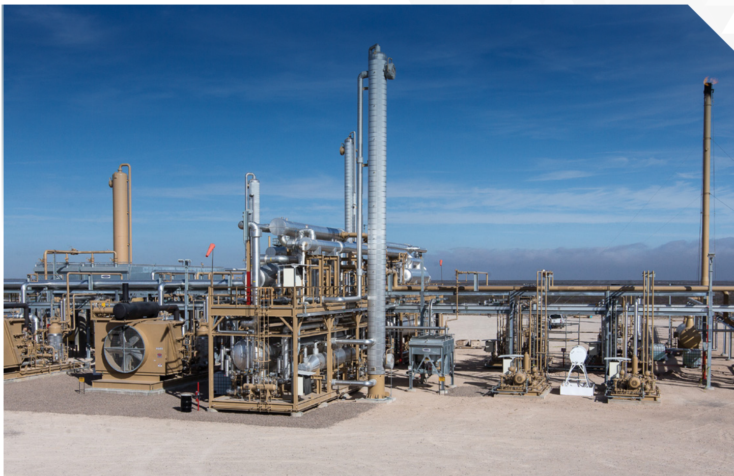
ITK gas plant with a combined design capacity of 450 mmscf/d of refrigeration and 410 mmscf/d of inlet compression, USA.
