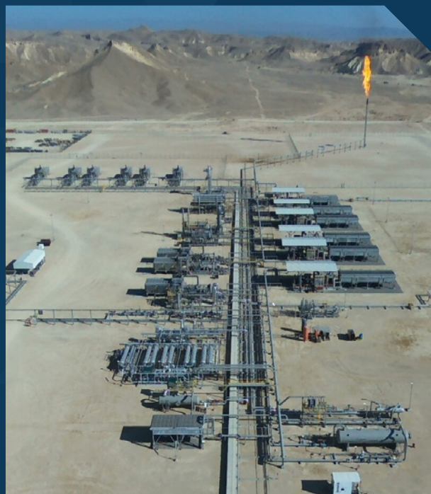
120 mmscf/d rental natural gas compression and processing facility, Oman.
